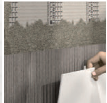
Tile laying using the thin-bed method. Apply tile adhesive COL-FLEX over the full surface using a notched trowel.
